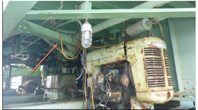
Aging Generator at Gwynn's Island Bridge
