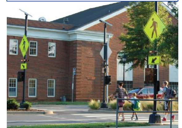
Rectangular Rapid Flashing Beacon
