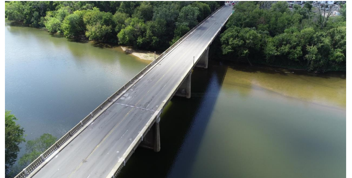
The Chatham Bridge was built in 1941, and is structurally deficient; It carries an average of 16,000 vehicles a day
