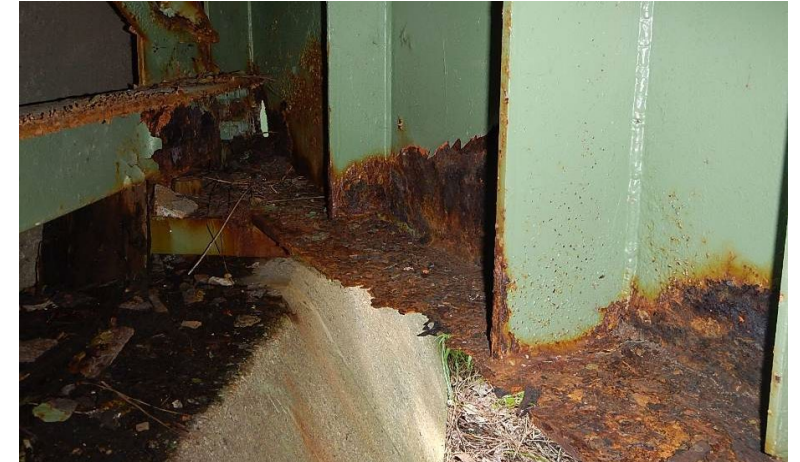
Poor (Structurally Deficient)
