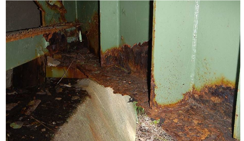
Poor (Structurally Deficient)
