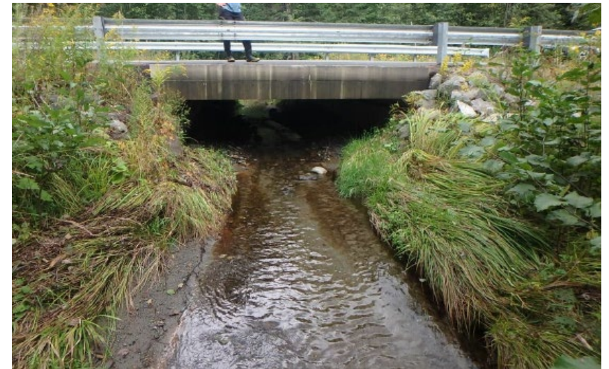
Box culvert with flat natural stream bottom providing fish and wildlife habitat values (USFWS).
